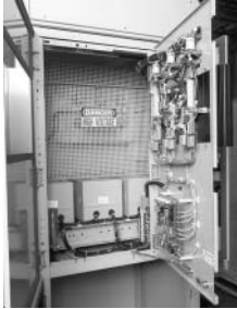
Mark V Field Controller
