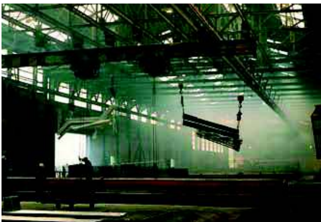
Feed and control of bridge cranes in a galvanizing plant
